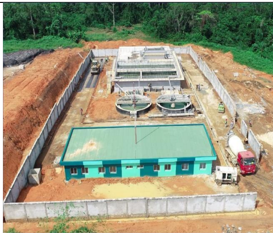
Image showing the site of the wastewater treatment plant at the Pk 24 Akoupé-Zeudji industrial zone
